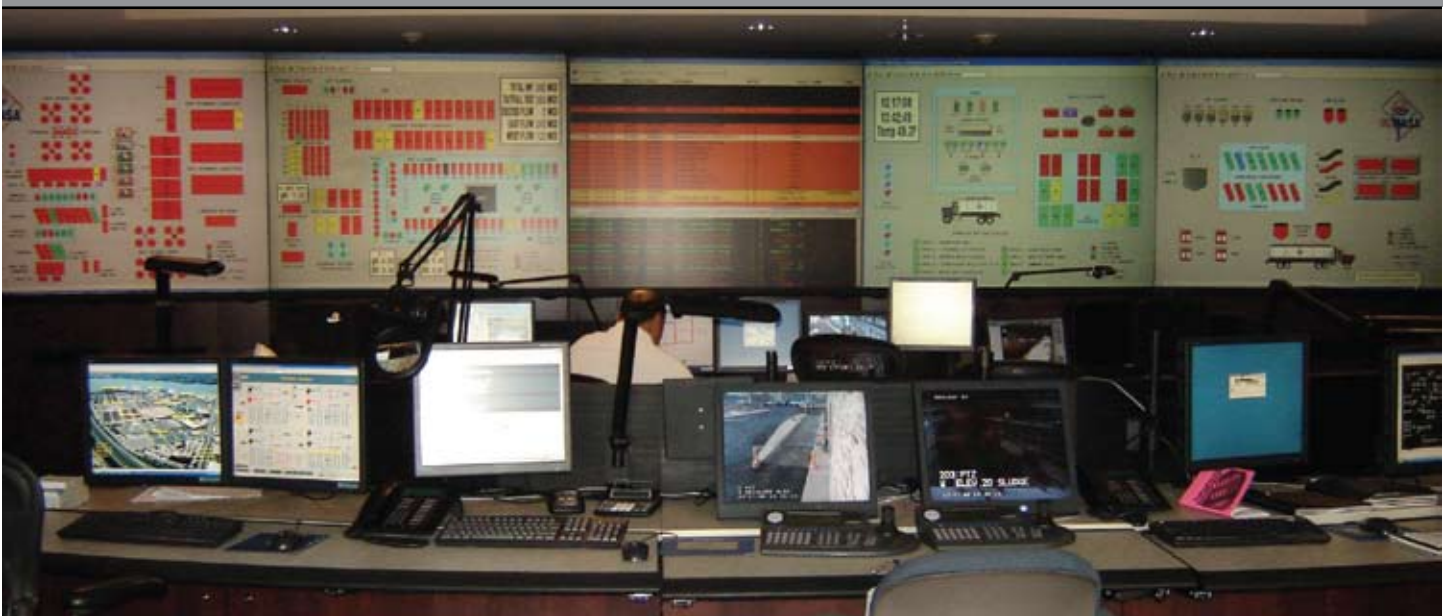
The Control Room is the heart of PCS at Blue Plains, serving as the centralized point of control for all of the facility's treatment processes.
